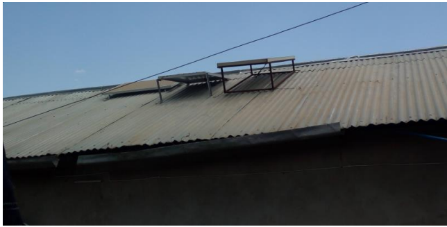
Fig. 1: Solar PVs mounted with different PV-roof spacing
