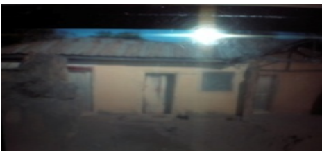
Plate 3: Building roofed in the Year 2004 showing Reddish- Brown Rust Spots
