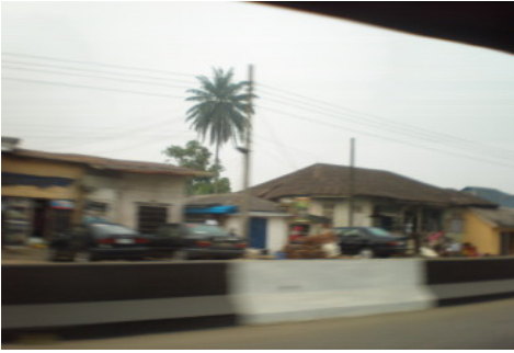
Plate 1: Buildings Close to the Main Road and Roofed in the Year 2001 had Shiny Roofs but have now (2013) turned Completely Reddish Brown
