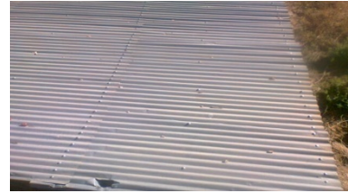
Plate 5: Building Was Roofed in Year 2010; Dulling of the Surface has Already Taken Place
