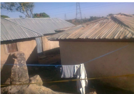
Plate 4: Two Buildings the First from the left was Roofed in Year 2007 and the Second Was Roofed in 2004. Rust has taken Away the Shining Beauty of the Second Roof
