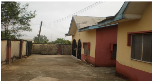
Plate 2: Building roofed in 2003 showing Light- Brown Rust Spot uniformly on the Zinc-plated roofing Sheets
