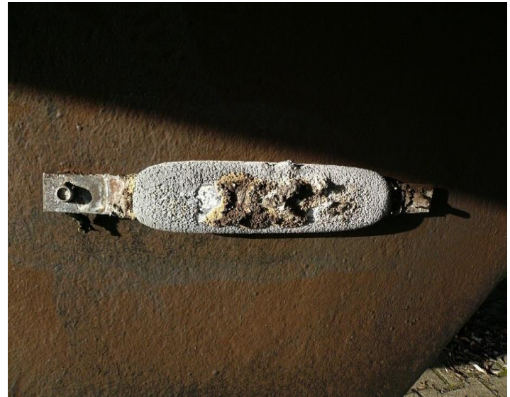
Fig 14: A deteriorating sacrificial anode
