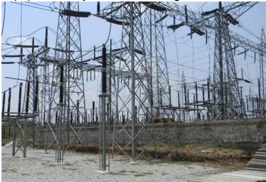
Fig. 1 A 220 kV substation in Mysore, Karnataka, India with different bay at different heights (Courtesy: KPTCL, Karnataka, India).
