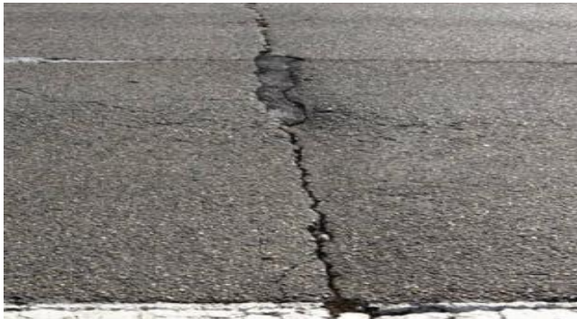
Fig. 2: Transverse crack on flexible pavement.
