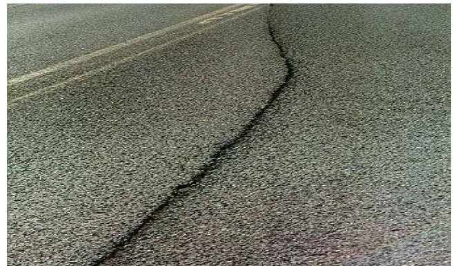
Fig. 1: Longitudinal crack on flexible pavement.
