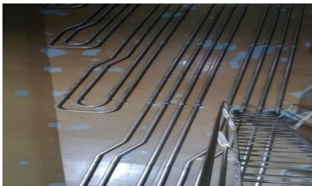
Fig. 2. SS heating coils and ladder in Chemical tanker tank (visible points of pitting repairs)
