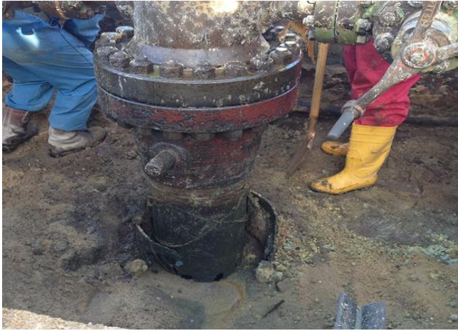
Figure 3: Corrosion and a big hole on 33.9725 cm casing
