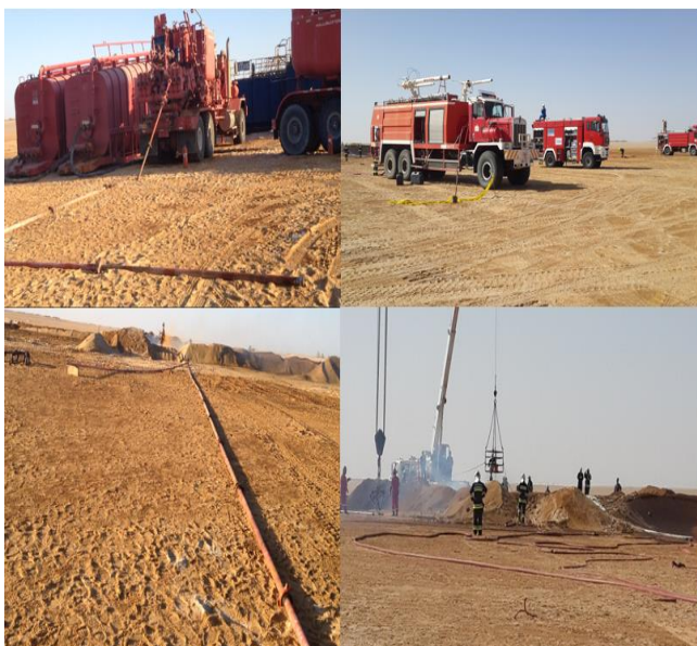
Figure 2: Rig up the surface line and Safety fire trucks with the crew standing on location 24 hrs for precaution.
