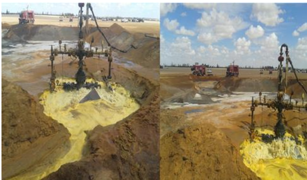
Figure 5: Wellhead with passageway killing fluid to the surface.
