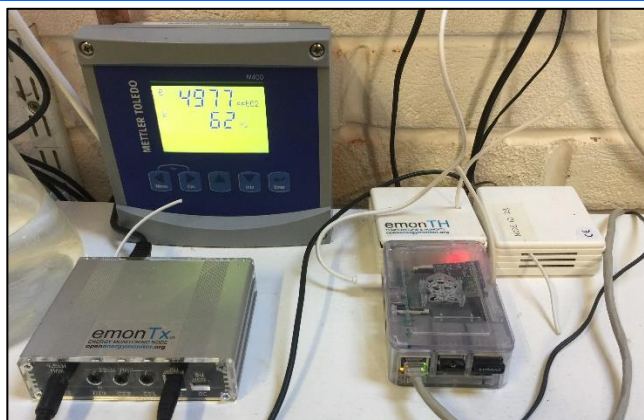
Fig. 2. EmonTX (front left), EmonHub (front right), Dissolved Oxygen Sensor (rear left), 2x EmonTH (rear right)
