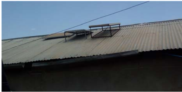
Fig. 1: Solar PVs mounted with different PV-roof spacing
