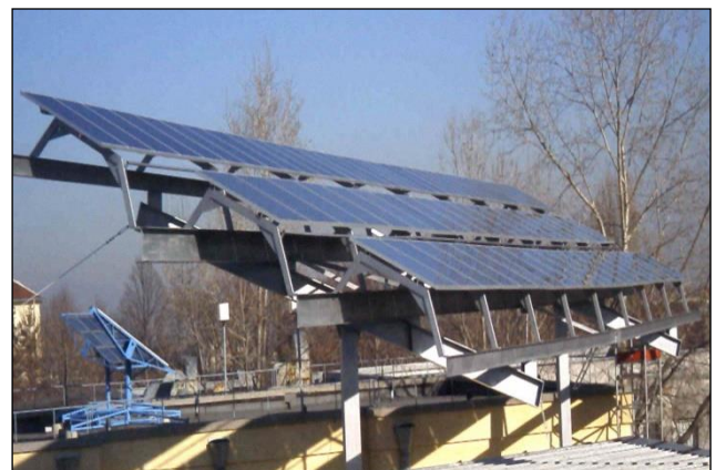
Fig.1. 10kWp PV rooftop - general view
