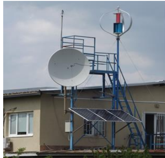
Fig.7. General view of hybrid (solar and wind) system for building application
