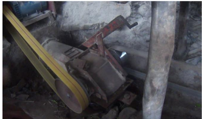
Figure 4.1 picture installed machine
