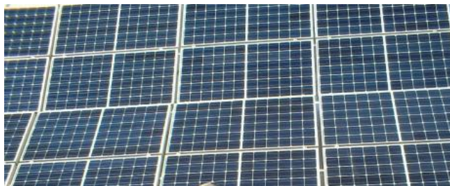
Fig. 4: Arrays of solar panels
