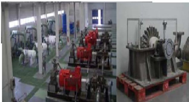
Figure 7: Tordera: the four groups(left one) and a dismantled Pelton turbine(right one)
