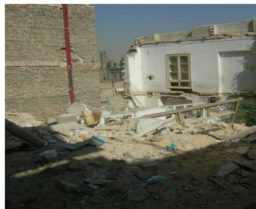
Fig. 2. Deteriorated area in Gheytrariyeh region
