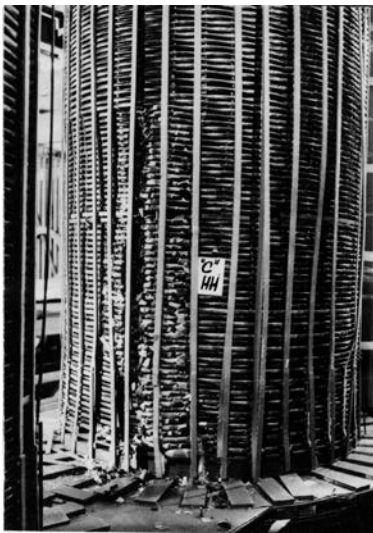
Figure 2. Typical example of deformation due to radial buckling in the C phase LV internal winding of 250 MVA /220 kV transformer ( \Delta X_k = +3,1\% ).
